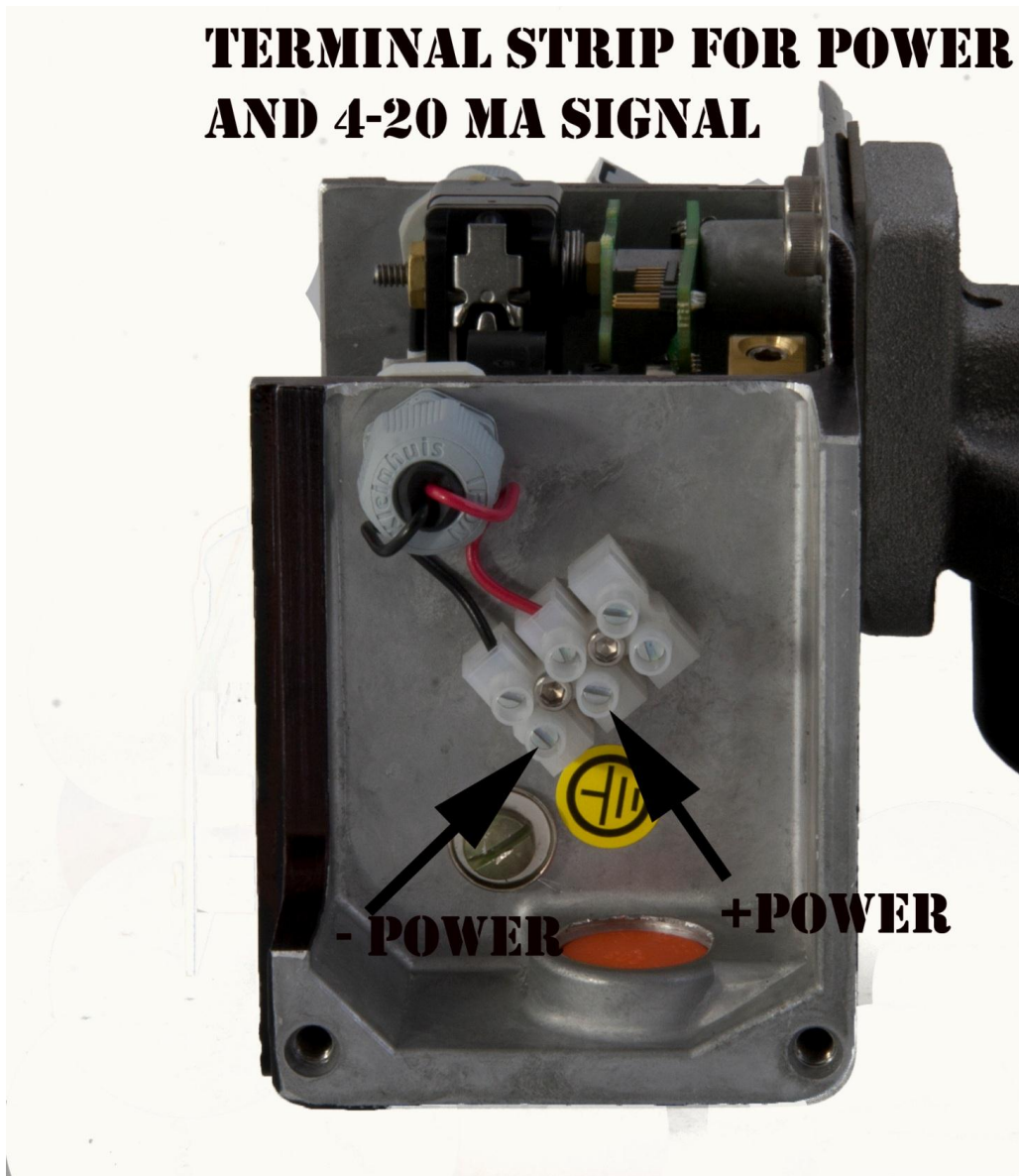
Figure 32: Terminal Strip for Power and 4-20 mA Signal
